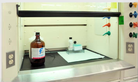
Engineering Control: Chemical Fume Hood
